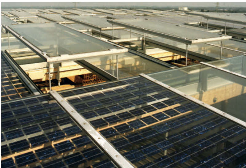
View onto the Roof of the Main Building of Revitalized Mining Facility
